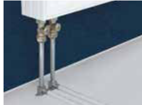
with connection valves
